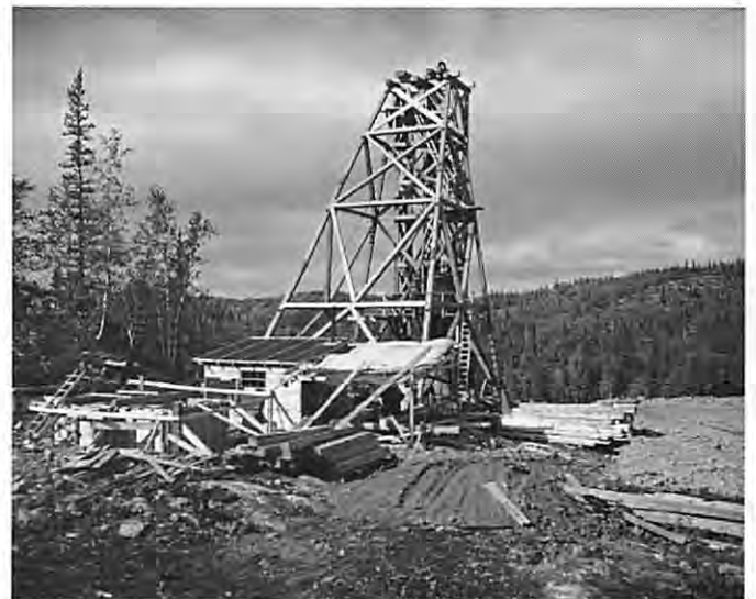
Head-frame under construction in 1949, at the Nicholson Mine (Courtesy of Glenbow Museum Archives. Photo NA-4510-30).
